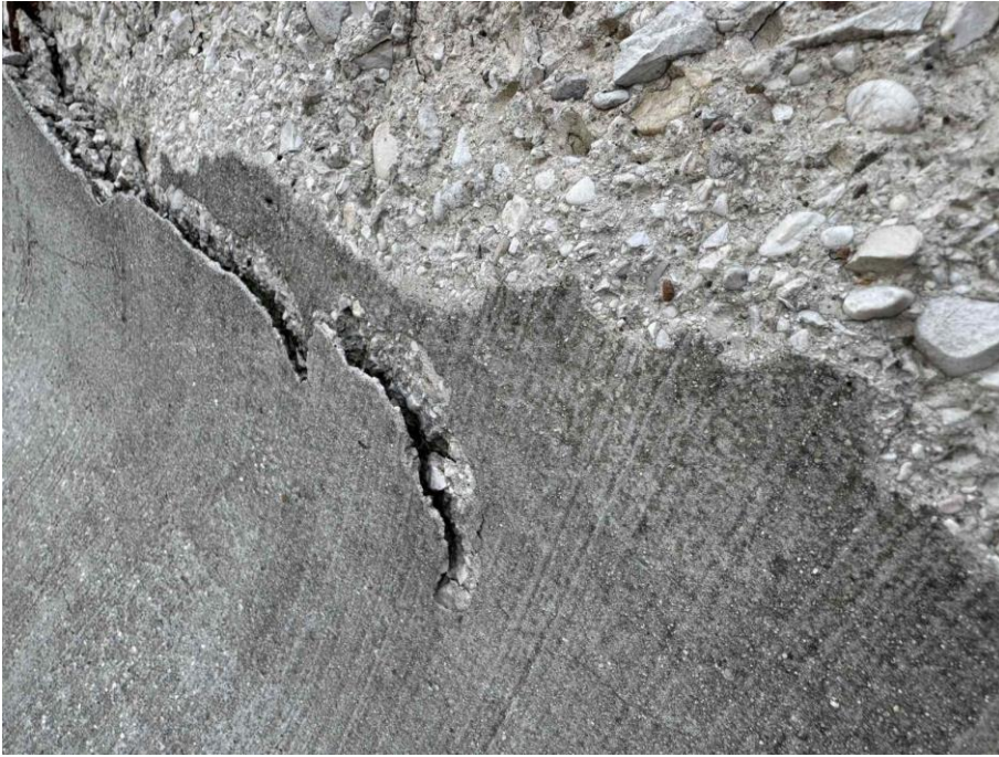
Figure 24 Diagonal cracking and edge separation caused by repeated vehicle contact and surface fatigue
