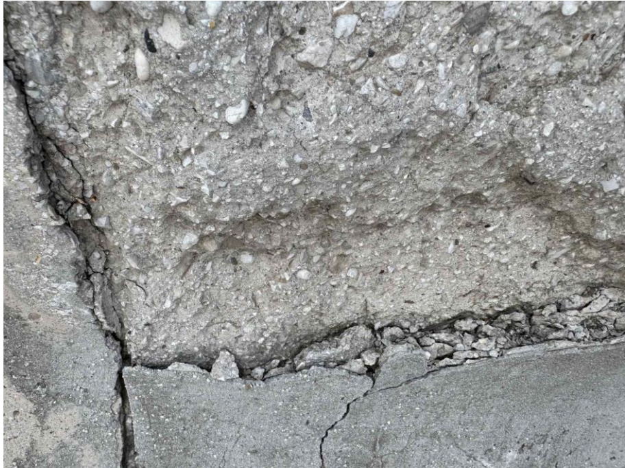
Figure 25 Cracking and minor joint separation suggest structural stress and possible construction-related defects
