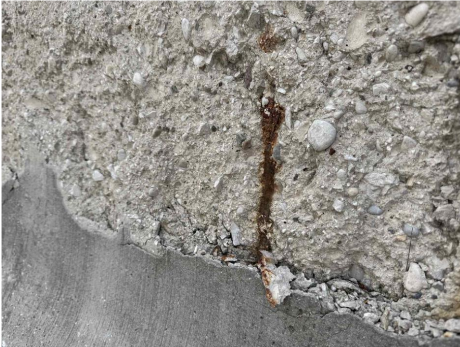
Figure 26 Evidence of corrosion-induced staining embedded steel reinforcement, indicating chloride ingress and carbonation
