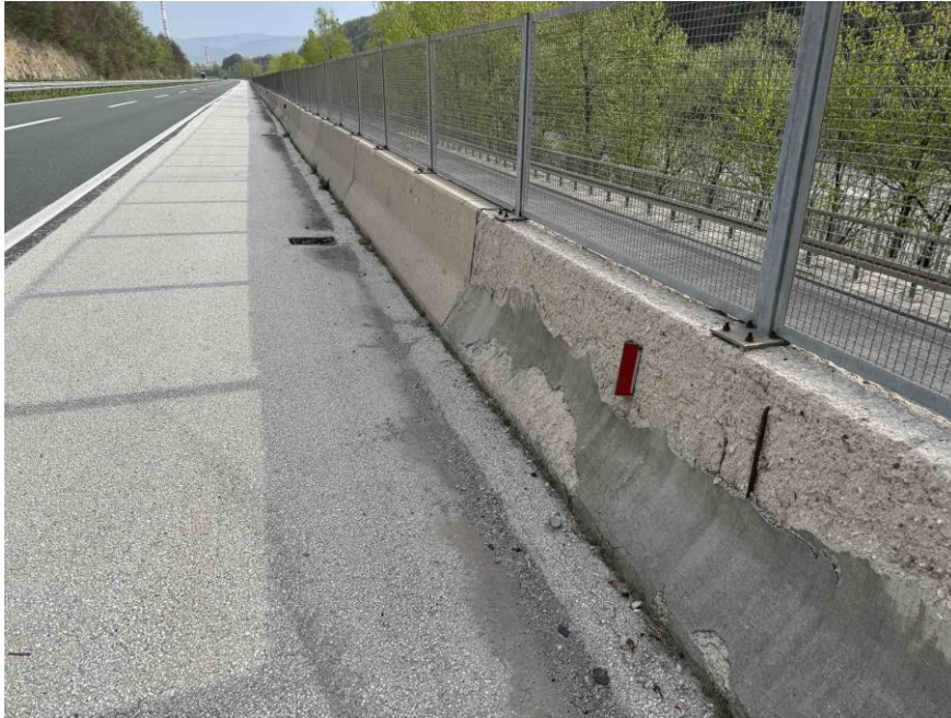
Figure 28 General view of deterioration New Jersey barrier showing large areas of spalling, surface scaling and reinforcement exposure near high-traffic segment
