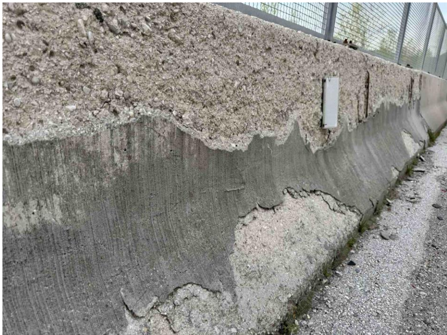
Figure 31 Widespread delamination and material separation likely due to inadequate surface treatment and poor curing
