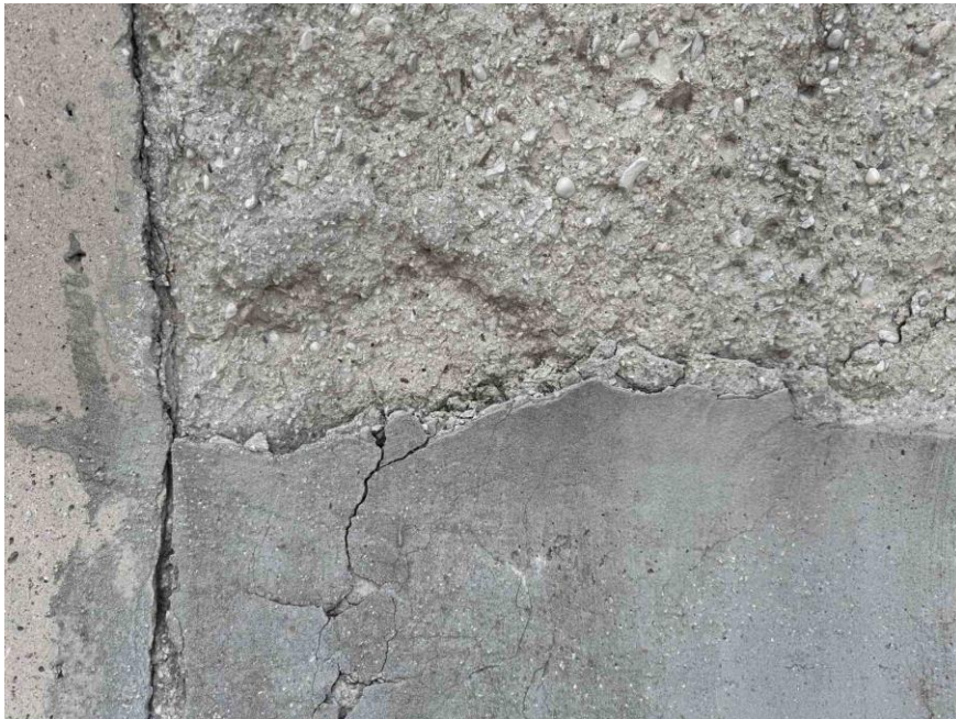
Figure 29 Vertical and transverse cracks along the lower section of the barrier, indicating structural fatigue and environmental wear
