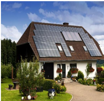
Figure 8: Solar panels on the roof of a family house [7]
