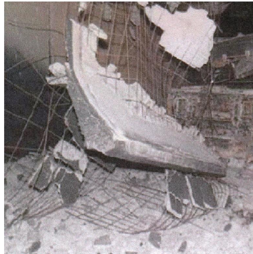
Figure 2. Damage of structure [5]
