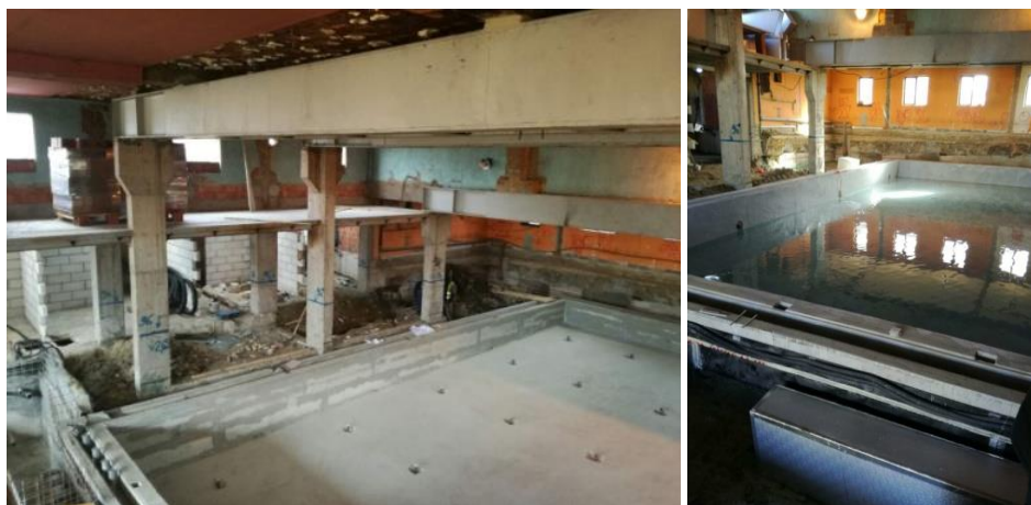
Figure 15. The inner part of the building with the newly designed structure and pool
